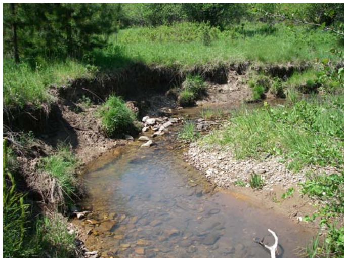
Eroding bank before restoration
